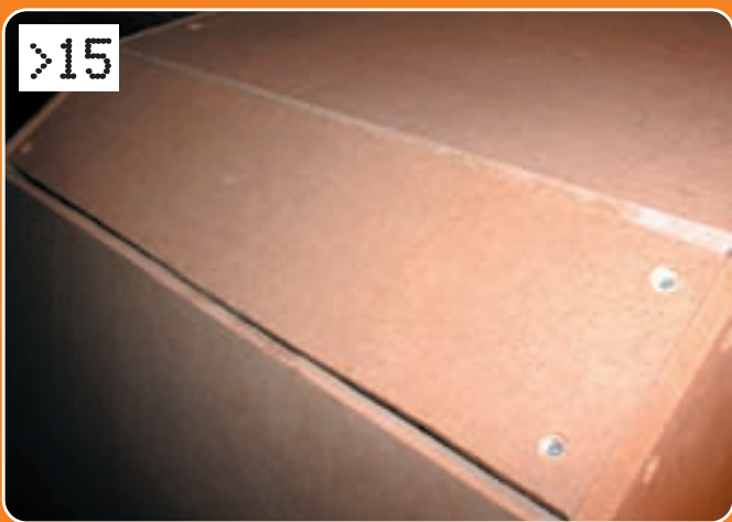
>15 Then it's time to add the rest of the roof, which again will be attached using batons screwed into the roof panels and the sides of the case. Competent woodworkers can mitre the edges of the panels so they fit snugly together; otherwise, keep the gap as small as possible so it can be filled later.
